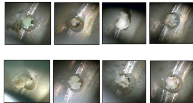
Figure 3. Blocked water separator drum holes.
